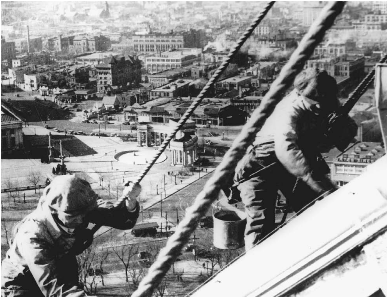
Men employed by the Civil Works Administration clean and paint the dome of the Denver capitol building in 1934. NATIONAL
