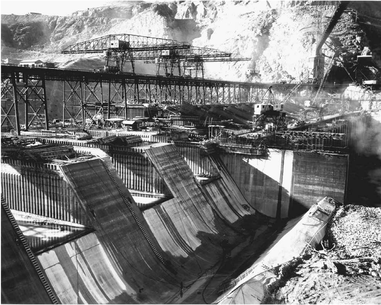
The massive Grand Coulee Dam, under construction in 1936 on the Columbia River in Washington. LIBRARY OF CONGRESS, PRINTS & PHOTOGRAPHS DIVISION, FSA/OWI COLLECTION
